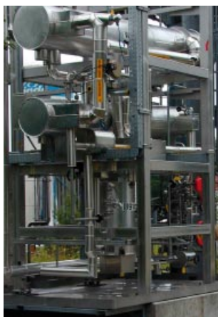
View of a cryo condensation plant
