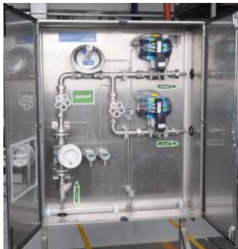
Figure 16: Complex measuring and metering station for nitrogen intended for the inerting of vessels, mixers and reactors [4]
