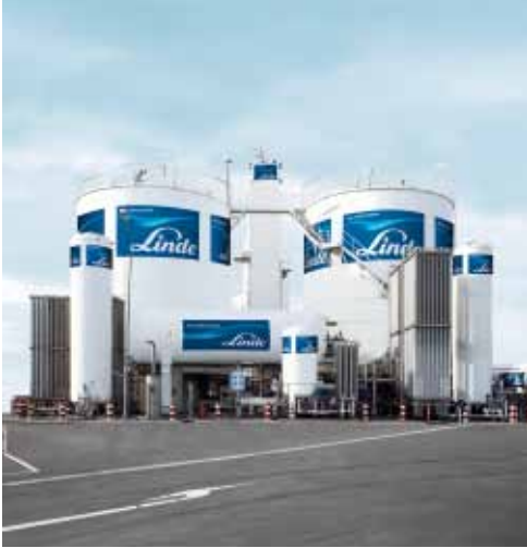
Figure 4: Cryogenic air separation plant
