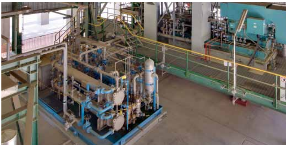
Figure 6: Small membrane separation plant
